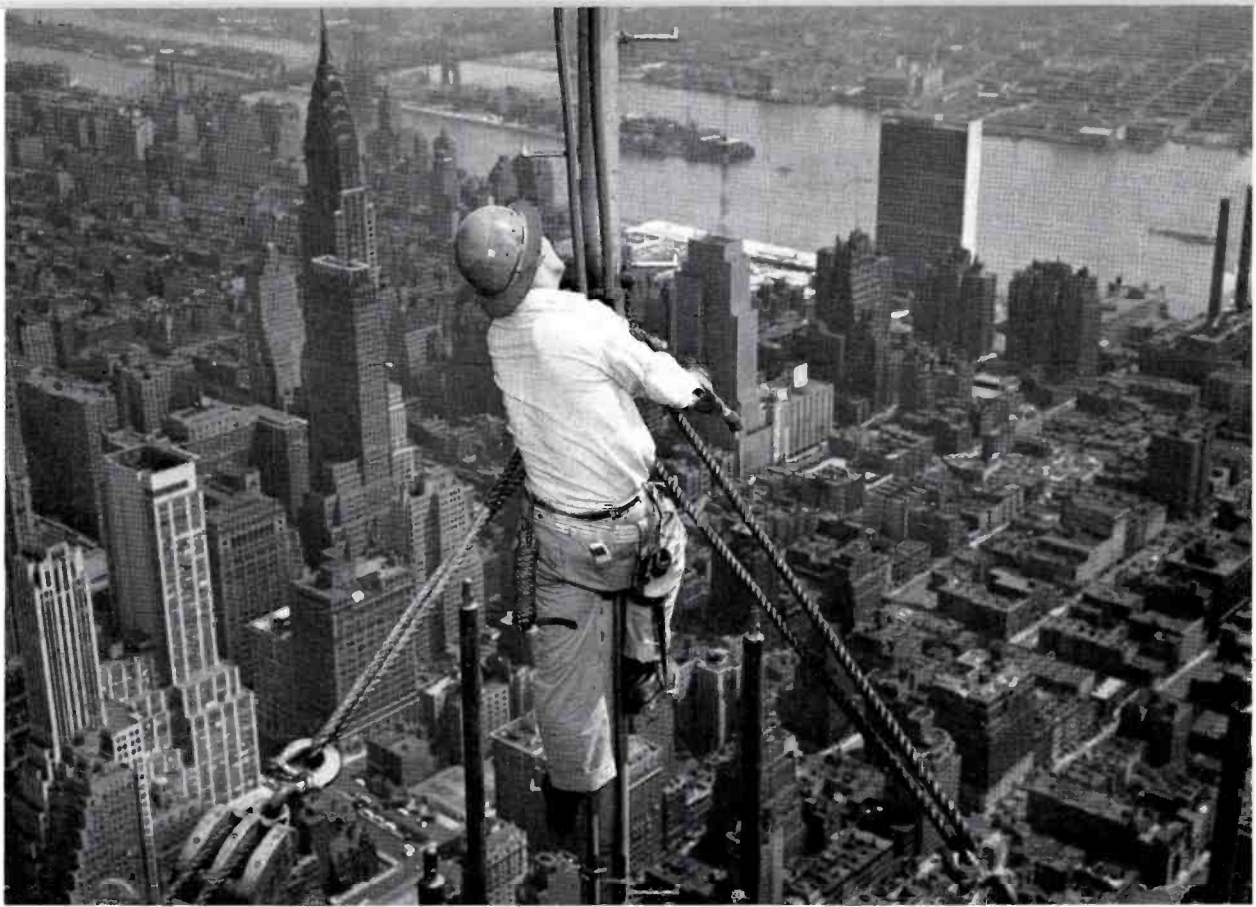
FIG. 2 (above). In this photo, Ray Corbet, American Bridge Company foreman, fastens lines to the 75-foot NBC temporary antenna which towers above: (left to right) the Chrysler Building with WCBS-TV antenna, Daily News Building with WPIX tower and the United Nations Building.
