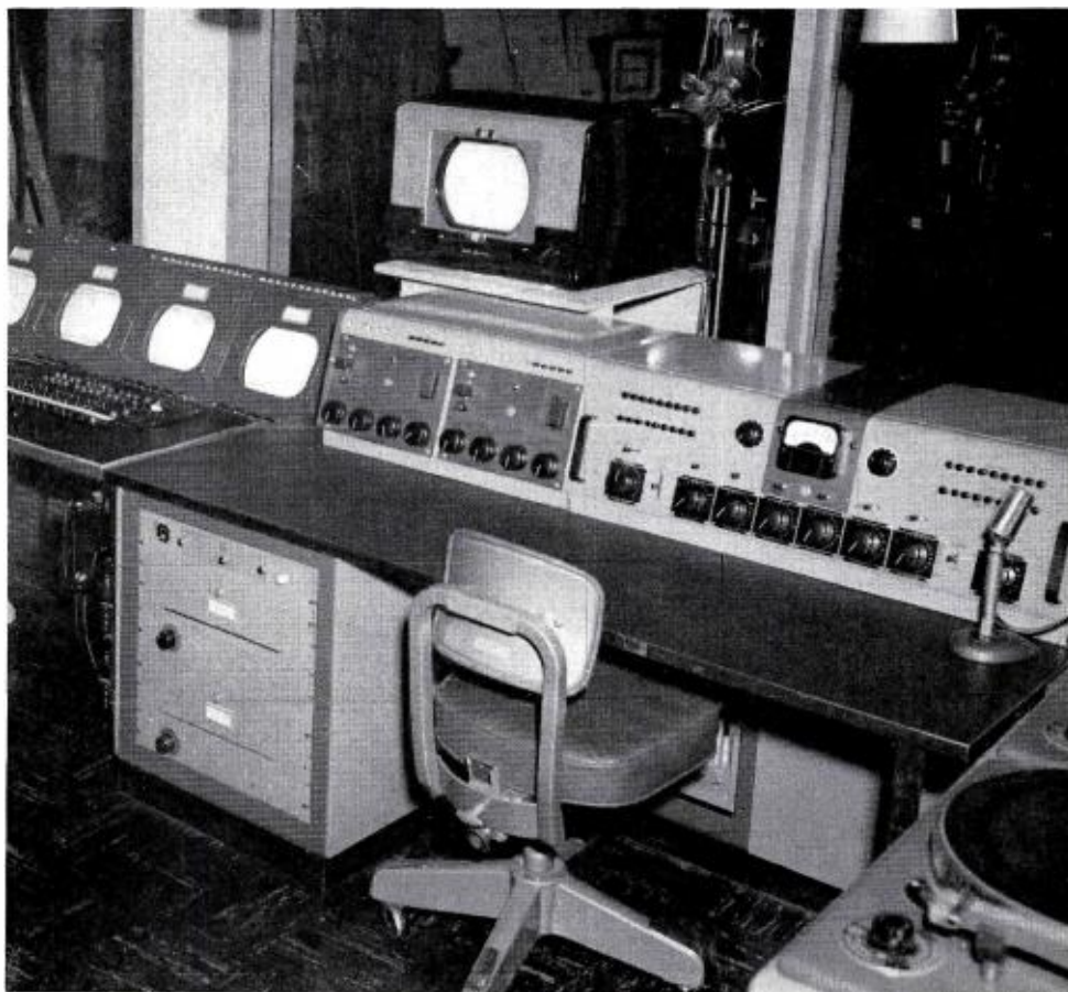
FIG. 20. Partial closeup view in studio "B" control room showing the audio control setup. Facilities consist of an RCA 76-B Console which is supplemented by two RCA OP-7 Mixer Amplifiers.
