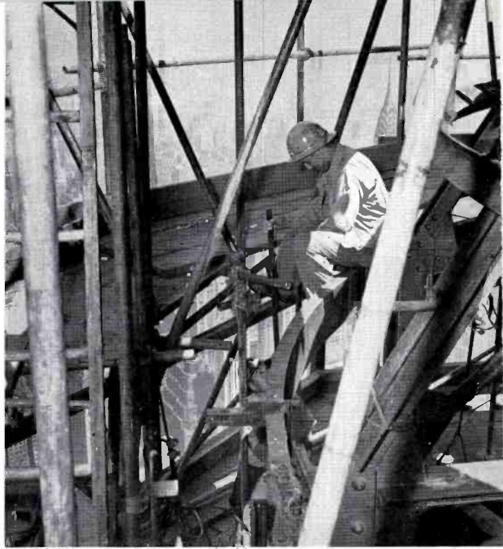
2 A three-story scaffold erected atop the Empire State building was necessary to provide adequate working space. Here, steel workers are shown completing the top working level, 1300 feet above the street level.
