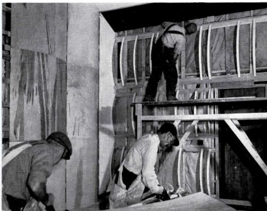
Studio B pictured during installation of acoustical treatment Roll insulation, the cylinder forms and fibre-covered cane ribs at right were covered with finished cylinders as shown at left.
