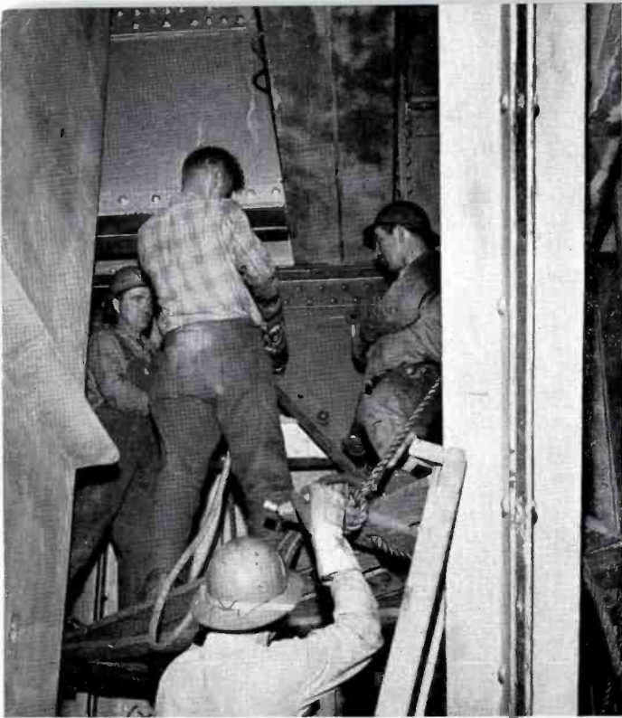
1 Here at the 96th floor, American Bridge Company steel workers are fastening new steel reinforcements to provide additional strength to accommodate increased activity, loads overhead, and the future 217-foot tower.
