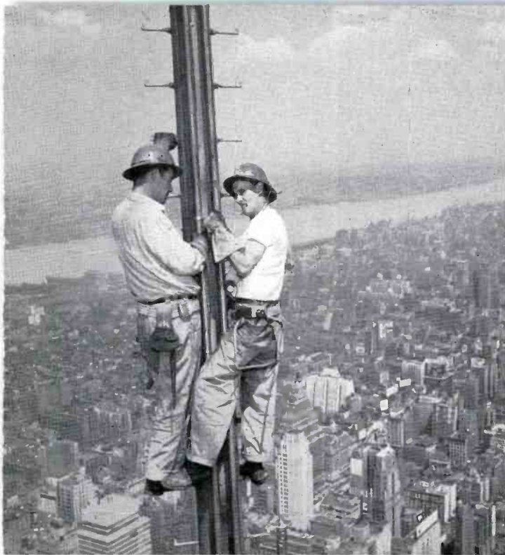
3 Before dismantling of the old TV antenna began, temporary antennas were erected to insure continuous service. Pat Corbet (right), 57, and son, Joe, 32 years old, are fastening transmission line on NBC's temporary antenna.
