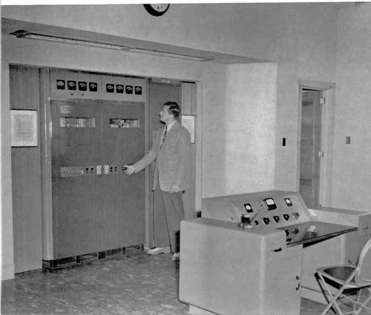
Left: WBRE-FM transmitter room. The RCA FM-1-C transmitter is built into the inset wall. Monitoring and test equipment is mounted on a rack just to the right of the transmitter. The convenient, streamlined control console was built by the WBRE staff. Shown in this view is Mr. David Baltimore, assistant manager of the station. He is the son of Louis G. Baltimore, owner and general manager of WBRE .
