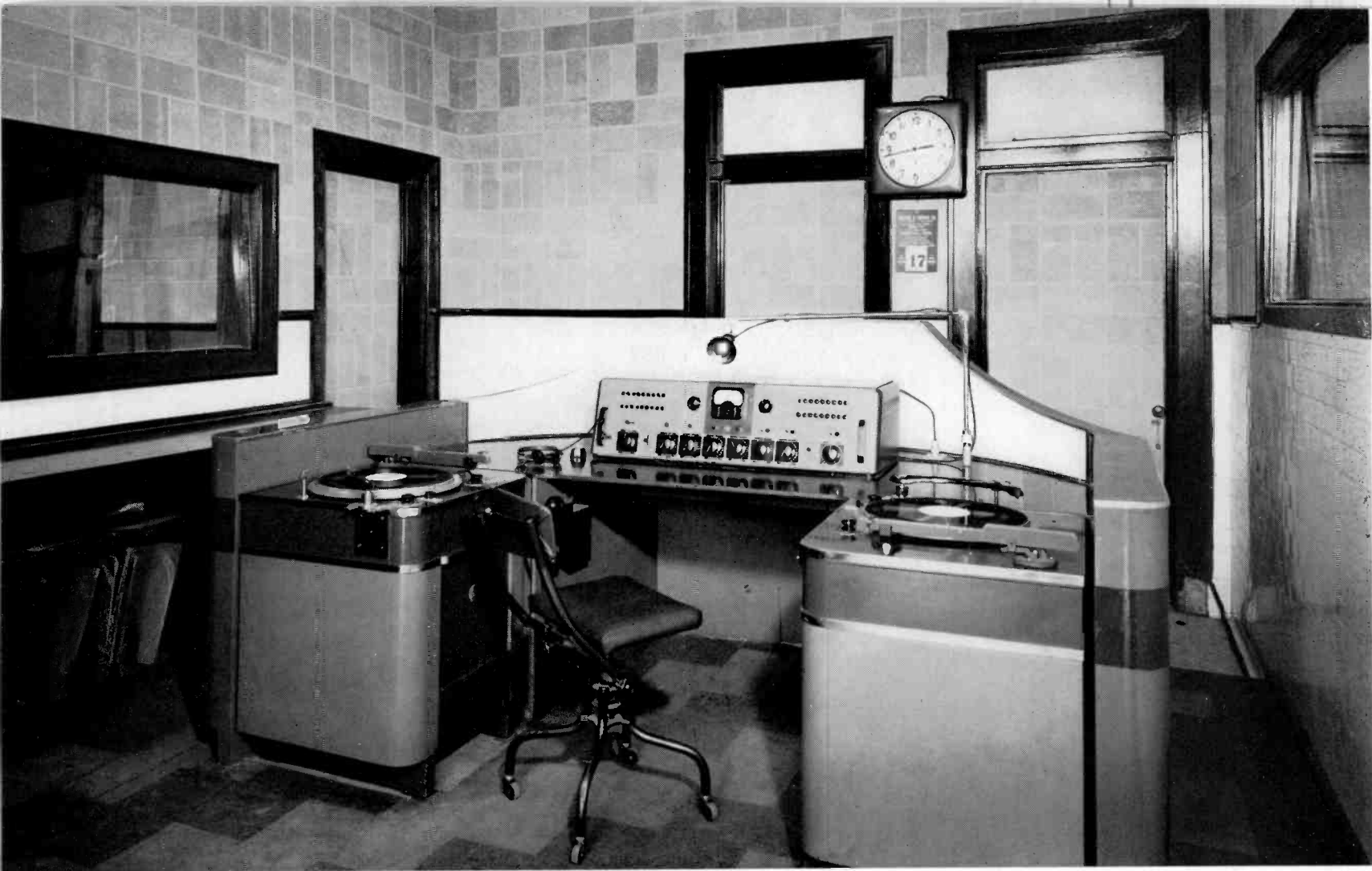
FIG. 1. (Above) Control room of WMOX. The streamlined control console, built by WMOX, has several ingenious features, including a guard wall, which protects the 70-C1 Turntables, an acoustic baffleboard behind the 76-B2 Console, and an 88-A Microphone mounted on a conveniently adjustable pipe-arm.
