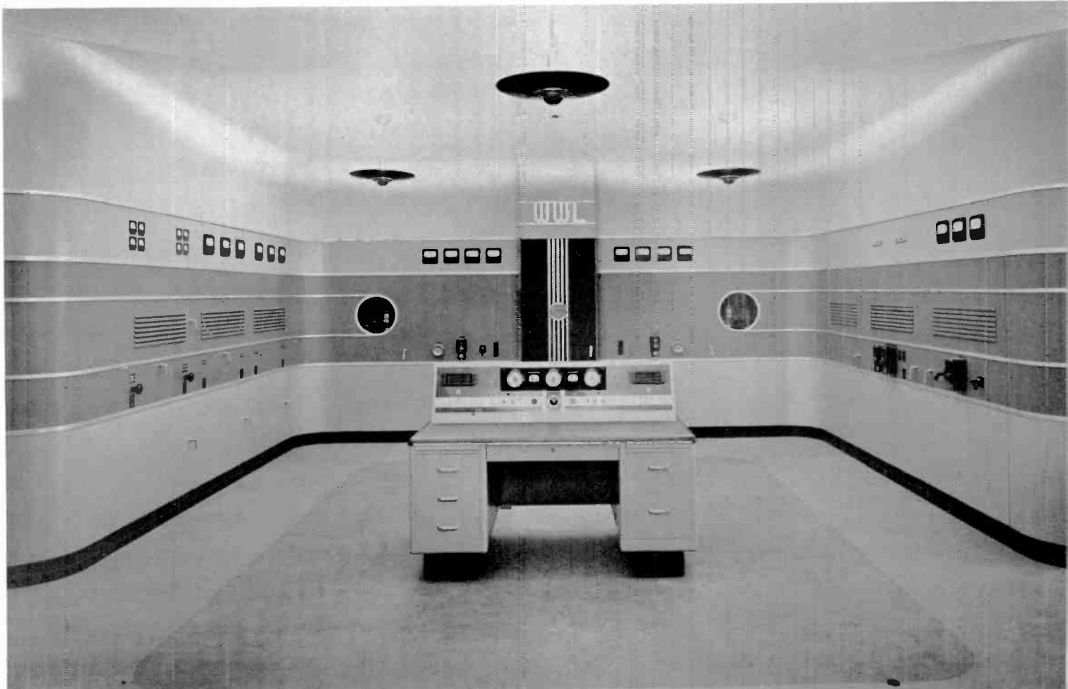
1938 WWL's fifty kilowatt RCA transmitter (shown below) was installed in a new building (see above) at a new site in 1938. It is one of the country's finest installations.
