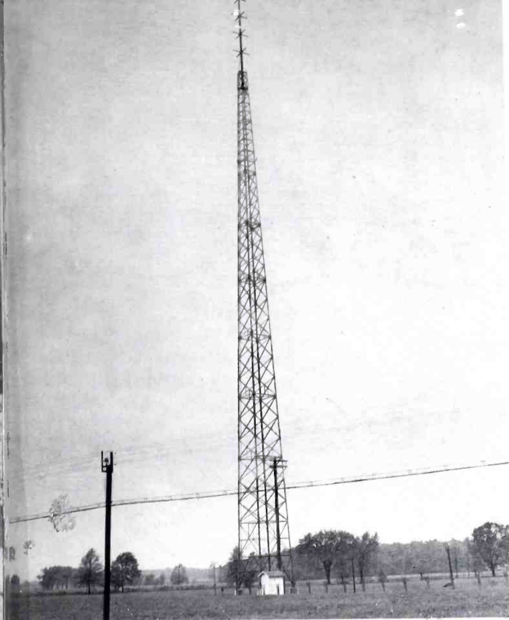
FIG. 8(c). ON AN AM TOWER. FM antenna of WSBF mounted on one of the towers of AM station WSBT, South Bend, Ind.
