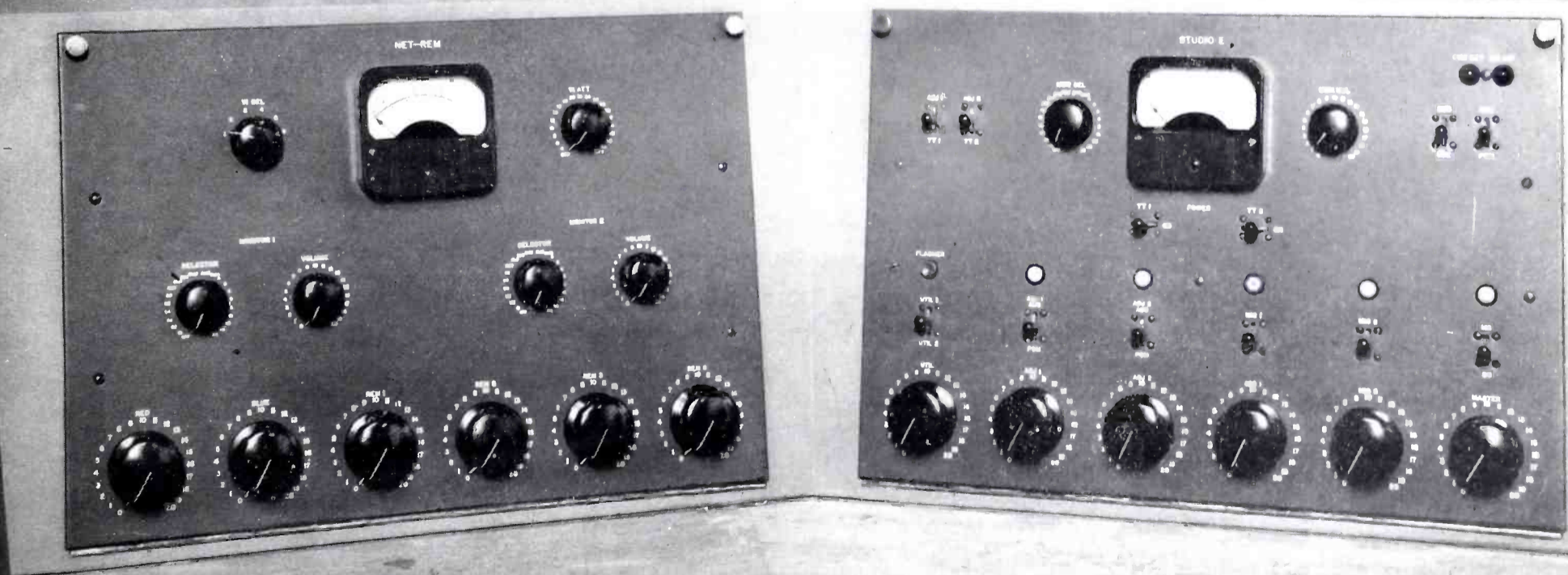
(Above) NET-REM and Studio E control panels on right side of desk.
