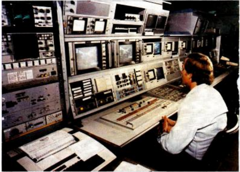
Master Control is an integral part of KCPQ's Technical Center. Machine controls and live and film camera video controls are built into the MC console.
