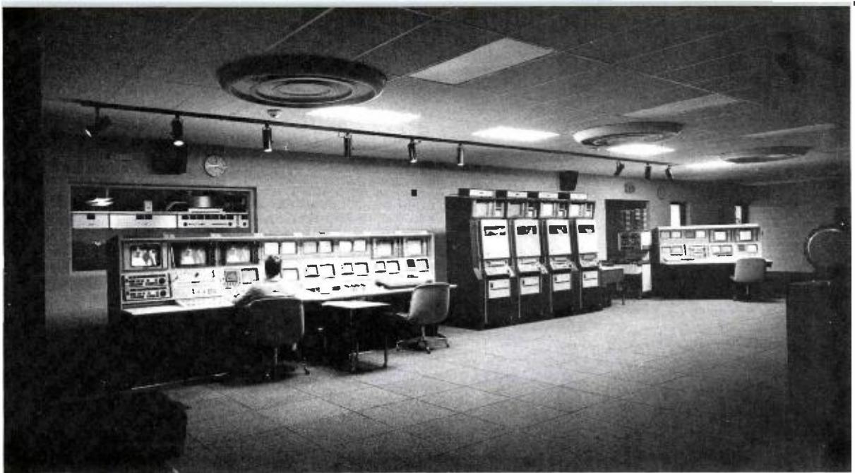
WCLQ-TV Technical Center is a spacious and amply equipped facility.
