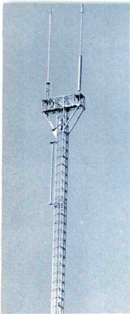
Three-antenna array atop Milwaukee's "T-Bar" tower includes a UHF Type TFU-36JDAS Pylon on left; VHF TW-12A Traveling Wave on right, and Pylon TFU-28DAS side-mounted on tower below the "T".
