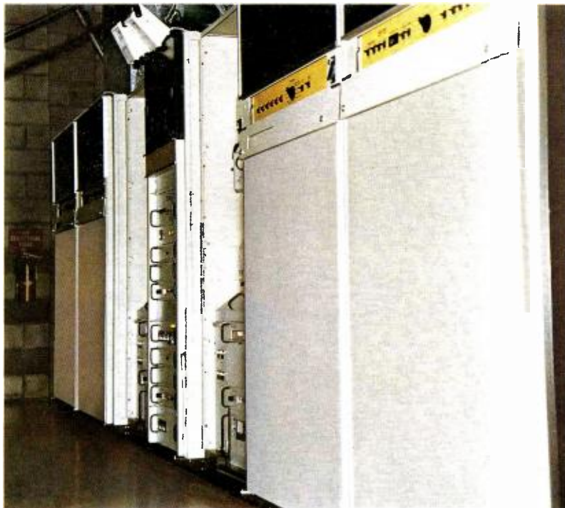
TTG-30/30H Transmitter is a parallel 60 kW system.
