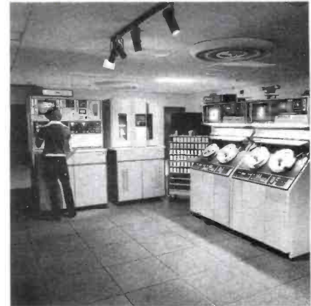
TR-600 quad VTR's are used for production and program playback; the video cartridge tape machine for airing commercials.
