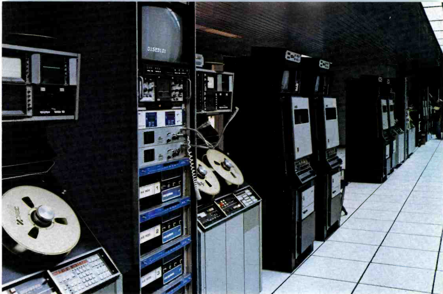
Extensive video tape capability is evident in this long line of VTR's at the Pacific Video Post Production Center.
