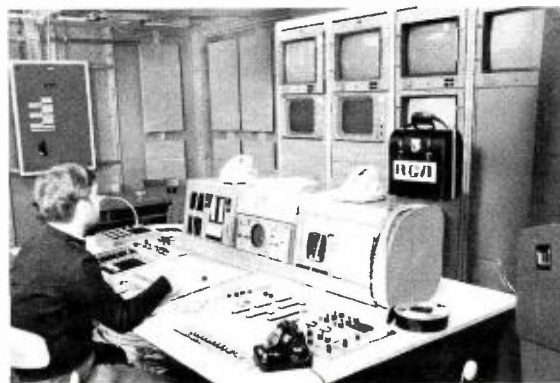
VTR mixing console with full remote control for all machines.
