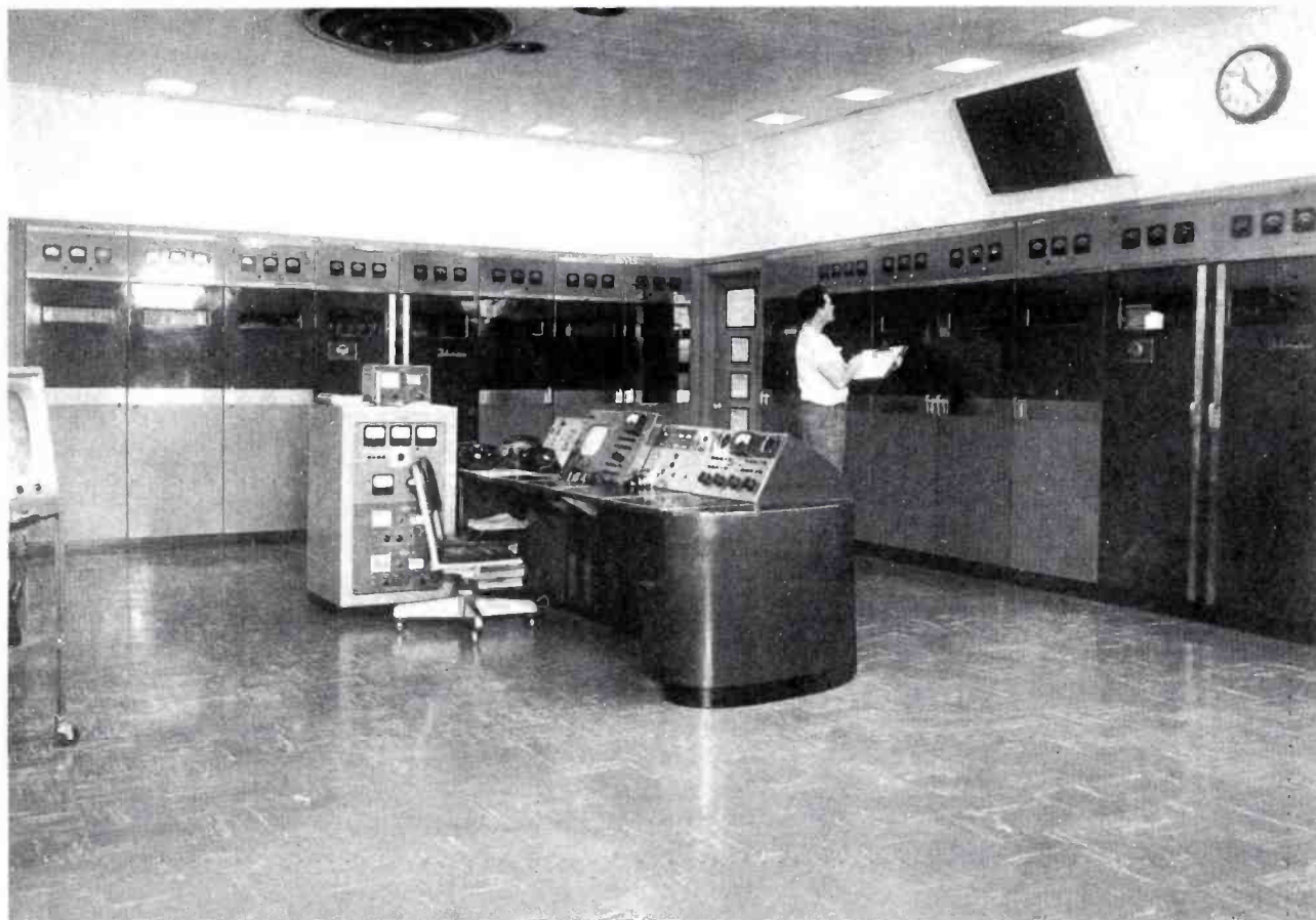
The two new 30 kW TT-30FL transmitters occupy less floor space than the TT-25 and TT-5 which they replaced. This "bonus" space in the photo above is being refurbished and will be occupied by the video tape operation which is scheduled to move from typically cramped quarters next to Master Control.
