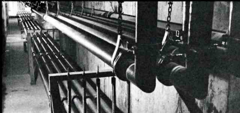
NEATLY ARRANGED AND CAREFULLY SUSPENDED, transmission lines are routed to assigned transmitter rooms.
