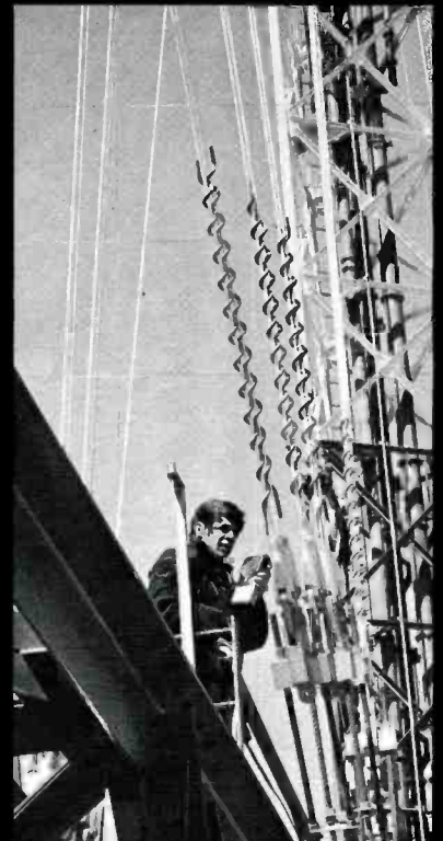
STANDBY TRANSMISSION LINE runs are contained in one tower leg; main lines in the second, and an elevator in the third.
