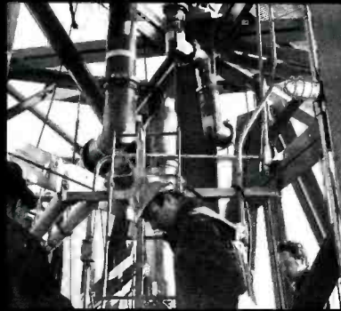
MAZE OF PIPES AND STEELWORK shown in this construction photo is indicative of the complexity of the system.
