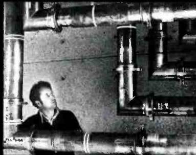
ELBOWS AND BENDS were a continuing concern for RCA engineer Ernie Baker during installation of transmission line.
