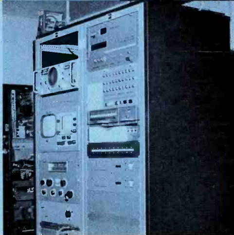
5 TT-50FH transmitter is equipped for remote operation, with a BTR-30 system (right) and automatic logging at the studio.
