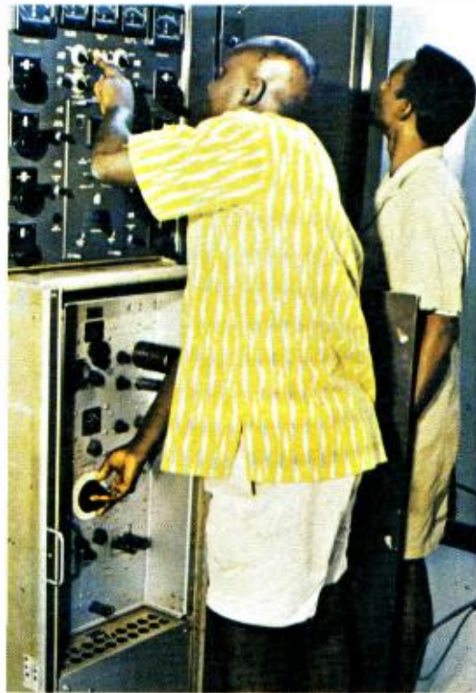
Radio transmitter exciter adjustment.
