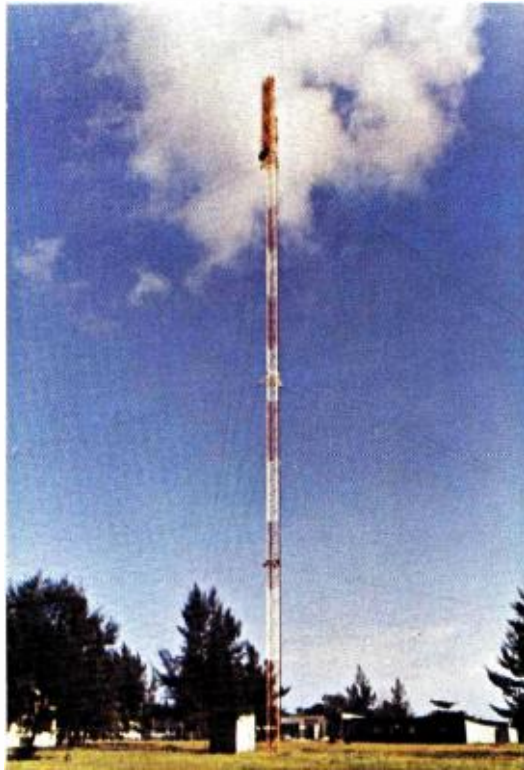
Antenna mast with microwave "Dish" for OB's.
