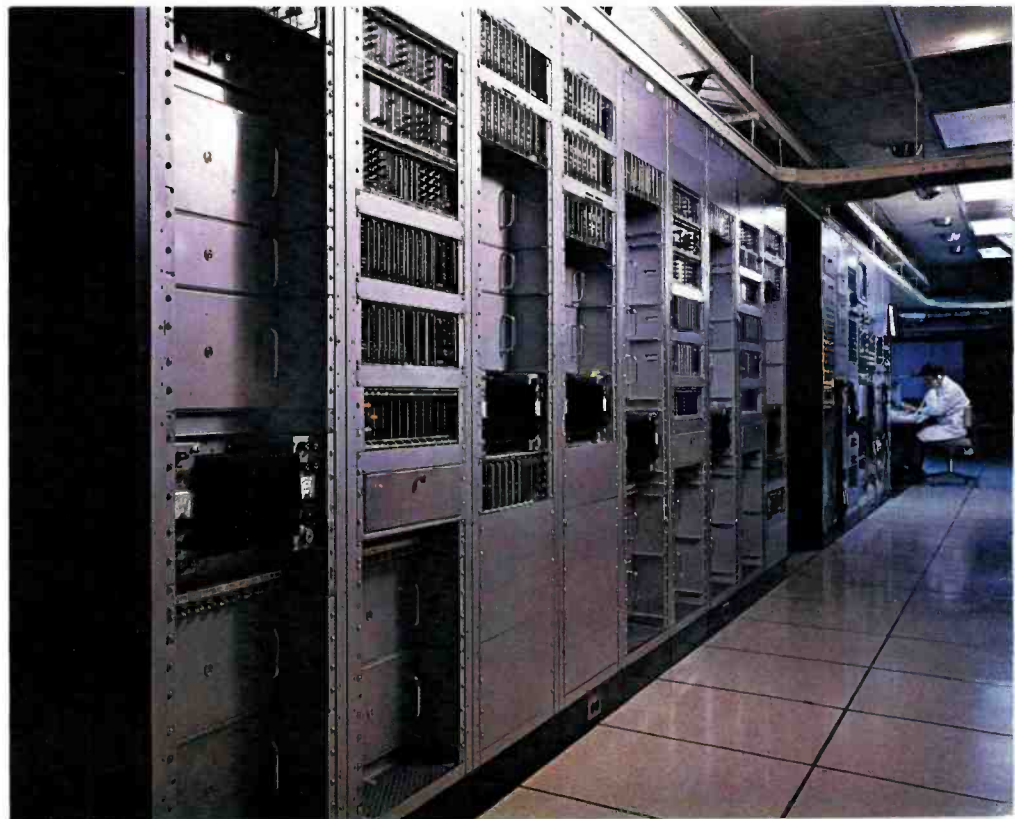
LONG VIEW OF VIDEO SWITCHING SYSTEMS looms large at the opposite end of OCR. Five TS-40 systems are housed here—assignment, Studio A, Studio B, master control, and house monitoring.
