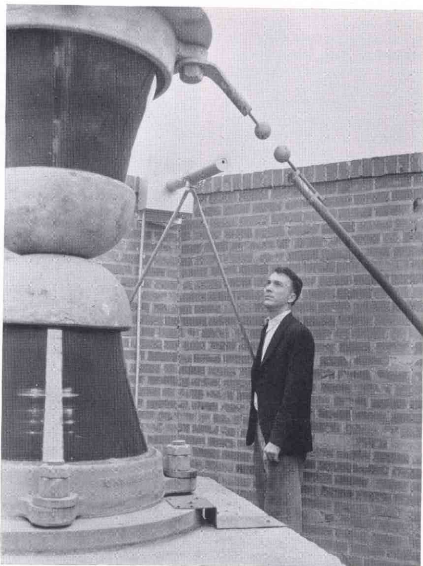
THE PHOTO-ELECTRIC "ARC EXTINGUISHER"—SOMEWHAT RESEMBLING A MACHINE GUN—IS MOUNTED ON THE WALL BEHIND THE BASE INSULATOR SUPPORTING THE 831-FOOT WLW VERTICAL RADIATOR ANTENNA TOWER. "AIMED" THROUGH THE LIGHTNING PROTECTIVE GAP, IT PICKS UP THE LIGHT OF ANY DISCHARGE AND PREVENTS POWER DRAINAGE BY MOMENTARILY INTERRUPTING PLATE VOLTAGE TO THE TRANSMITTER. WITHOUT THIS DEVICE, AN ARC ACROSS THE GAP WOULD CARRY OFF FROM THE ANTENNA VIRTUALLY ALL OF WLW'S 500,000-WATT POWER—ENOUGH ELECTRICAL ENERGY TO FILL THE RESIDENTIAL LIGHTING REQUIREMENTS OF A CITY OF 150,000 POPULATION. THE PHOTRONIC CELL AND ITS ASSOCIATED RELAYS ARE MOUNTED IN A DOUBLE METAL BOX WHICH CAREFULLY SHIELDS THEM FROM THE STRONG RADIO FREQUENCY FIELDS AT THE BASE OF THE ANTENNA. THE PHOTRONIC CELL IS MOUNTED AT THE END OF THE "BARREL" OR LIGHT TUBE. THE POWER RELAY OPERATES DIRECTLY ON THE TRANSMITTER CONTROL CIRCUITS AND ALSO OPERATES INDICATORS IN THE TRANSMITTER BUILDING
