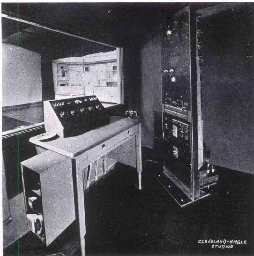
THE CONTROL ROOM OF THE WCAU AUDITORIUM STUDIO—COMPLETELY RCA EQUIPPED. www.americanradiohistory.com
