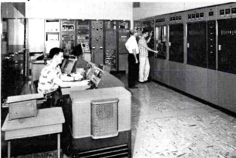
▼ FIG. 5. Television transmitter room showing 25 kw RCA Transmitter (used in conjunction with 12 bay antenna for maximum power).
