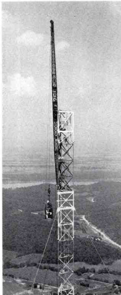
FIG. 4. At the site, 30-ft. sections were assembled and painted on the ground then hoisted aloft and bolted into place. Special hoisting equipment used consisted of a heavy boom (gin pole) that "walked" up the tower as it grew.
