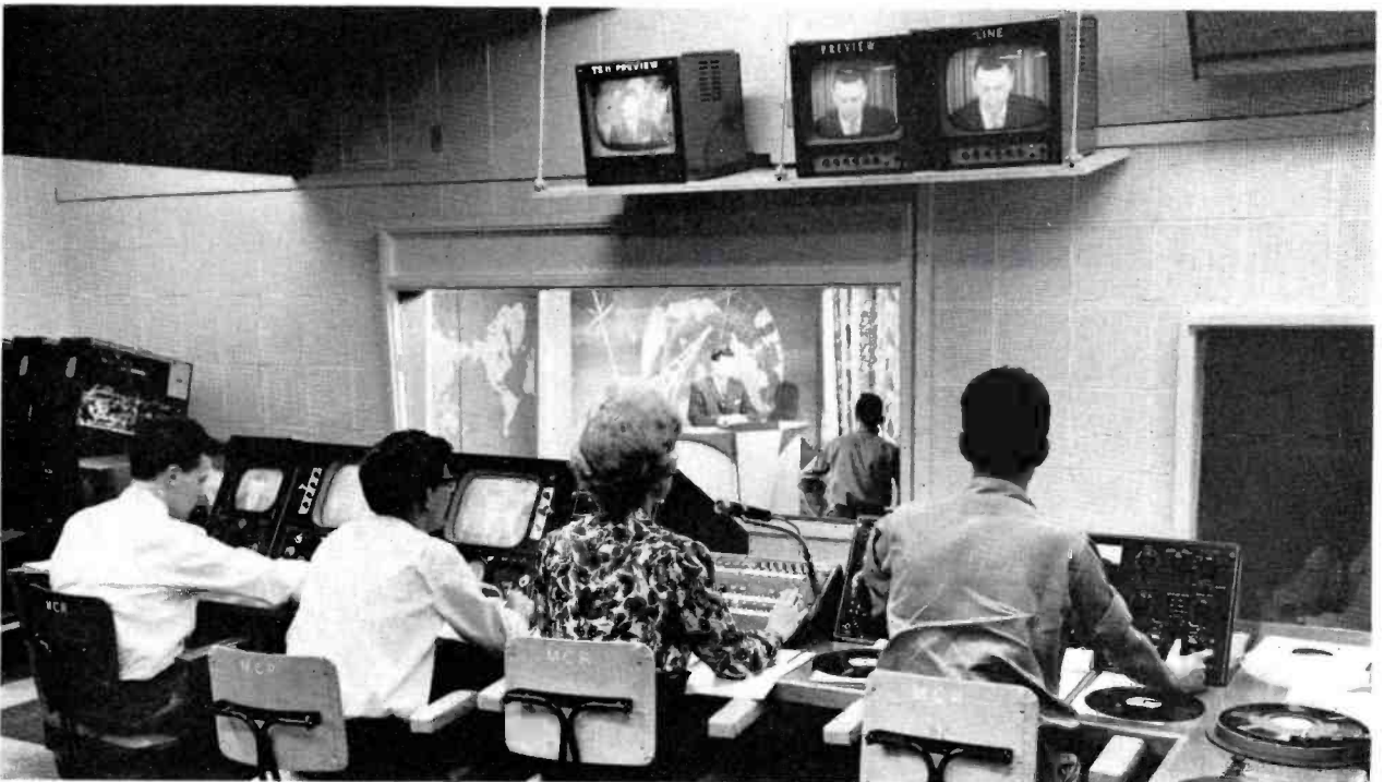
FIG. 12. Master Control serves a three way function as Studio C control room, transmitter control room and master control room. The RCA TS-40 switcher and BC-6B audio console provide flexible programme control facilities.
