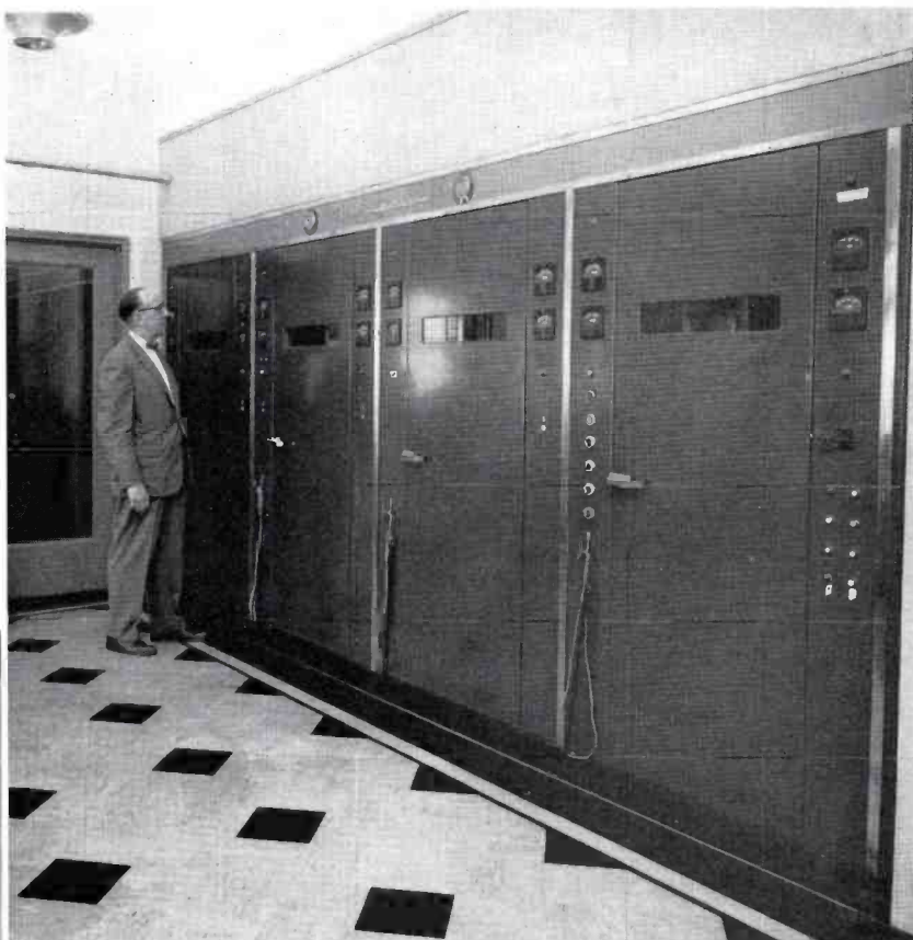
FIG. 24. WGN uses BTA-50G 50 kw Ampliphase transmitter. (It occupies same area required by former 10 kw transmitter.) Radio transmitter is remotely controlled 24 hours a day. (Shown is G. William Lang, Chief Engineer, WGN Radio.)
