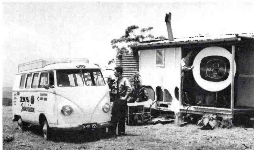
FIG. 17. A microwave link repeater station installed on Eagle Heights near the famous Gold Coast area of Queensland. This repeater station was being used to facilitate the telecast of the Rosebowl Tennis Tournament at Southport.
