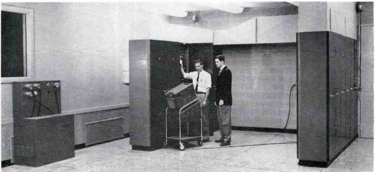
FIG. 18. Twelve racks with forced air ventilation are provided for the rack-type equipment. Space has been allowed for future expansion.
