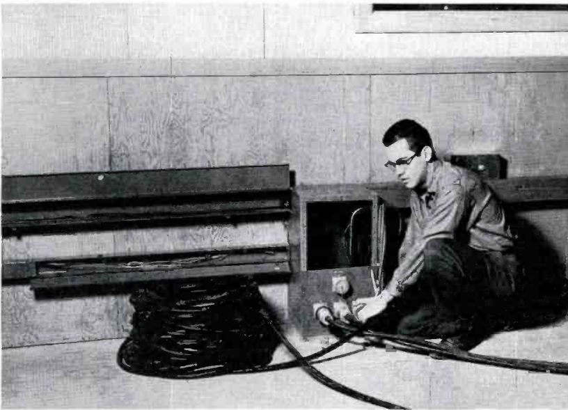
FIG. 8. Cables and wires can be terminated at any location in Studio A. Wireway with hinged covers circumscribe the studio; one is used for a-c power and the other for audio and video.
