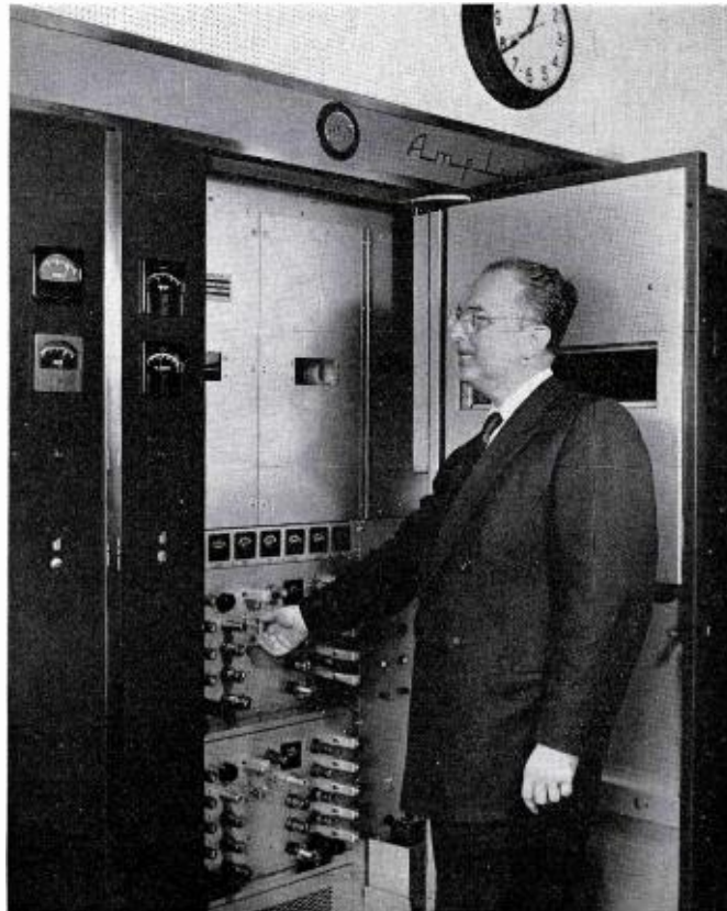
FIG. 1. Paul Von Kunits, WINS Chief Engineer, is shown making the one daily adjustment, the carrier level control, on the BTA-50G exciter modulator unit.
