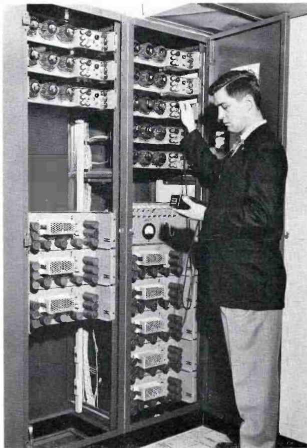
FIG. 17. Chief Engineer Jack Petrik at two racks which house power supplies for all 280-volt d-c requirements.
