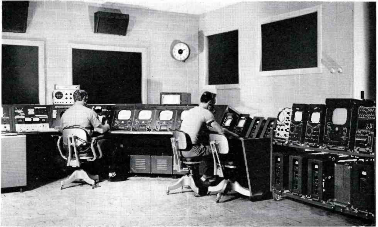
FIG. 13. Master control is located so that operator can see into both studio control rooms, both announce booths, and the projection room.
