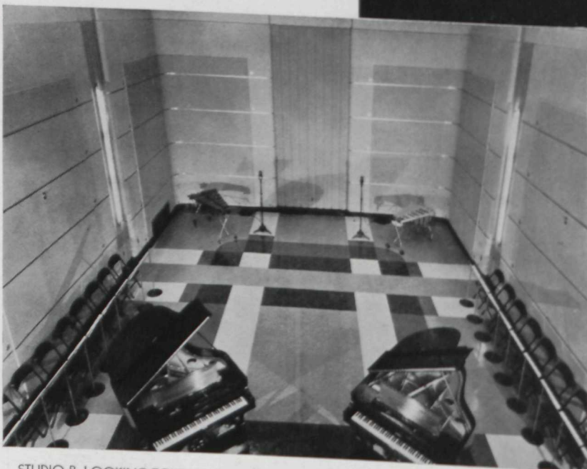
STUDIO B, LOOKING TOWARD THE "DEAD END." CONSIDERING THE BRILLIANT COLORS AND THE CHROMIUM METALLIC TRIM EMPLOYED IN THE DECORATION SCHEME OF THIS STUDIO, THE ABOVE VIEW IN BLACK AND WHITE HARDLY DOES JUSTICE TO THE SUBJECT.
