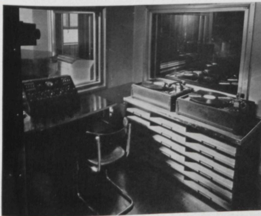
ELECTRICAL TRANSCRIPTION EQUIPMENT IN STUDIO H. THIS STUDIO IS A SPECIALLY AIR CONDITIONED CHAMBER DESIGNED TO PREVENT WARPING OF THE RECORDS IN THE METALLIC FILES AND TO INSURE UNIFORM PERFORMANCE DURING ALL ELECTRICAL TRANSCRIPTION PROGRAMS. THE AVERAGE PERSON DOES NOT REALIZE THAT FOUR PERSONS ARE REQUIRED TO HANDLE PROGRAMS OF THIS TYPE—ONE PRODUCTION MAN, ONE ENGINEER, ONE ANNOUNCER, AND A TESTING AND TIMING SUPERVISOR.
