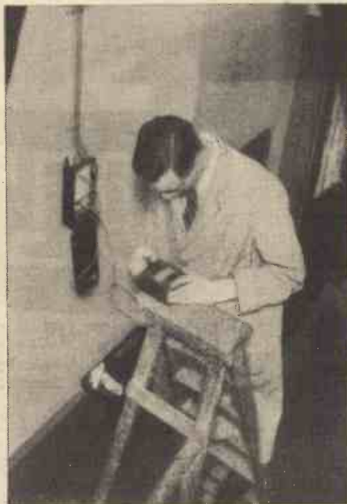
Testing a house-wiring installation for insulation resistance by means of a pocket-type "Megger"
