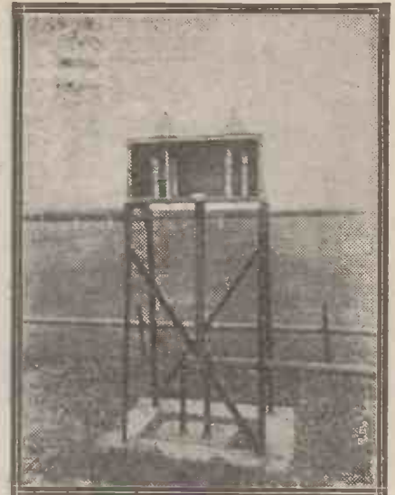
Another picture taken at the Bodmin Beam Transmitting Station, showing the box in which the aerial coupling coils are housed.
