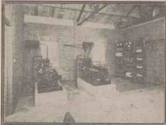
A view of part of the power house at the new radio station, showing the generators and switchboard for battery charging.
