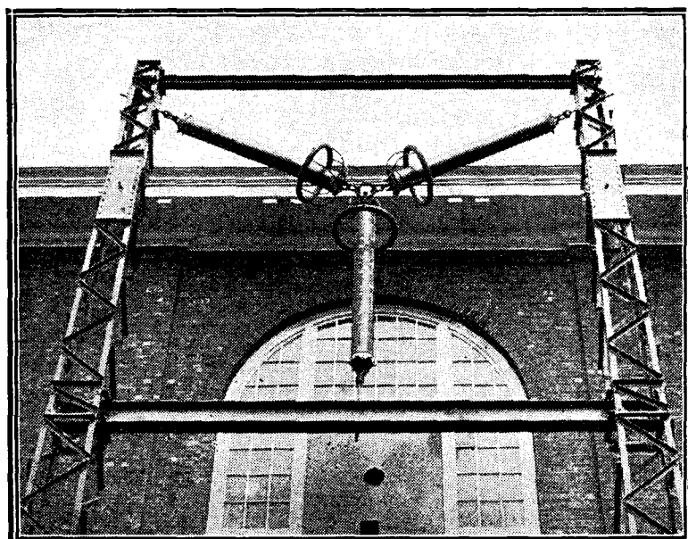
The "earth" lead-in at the Hillmorton Station, Rugby, is of very elaborate construction and very carefully insulated.
