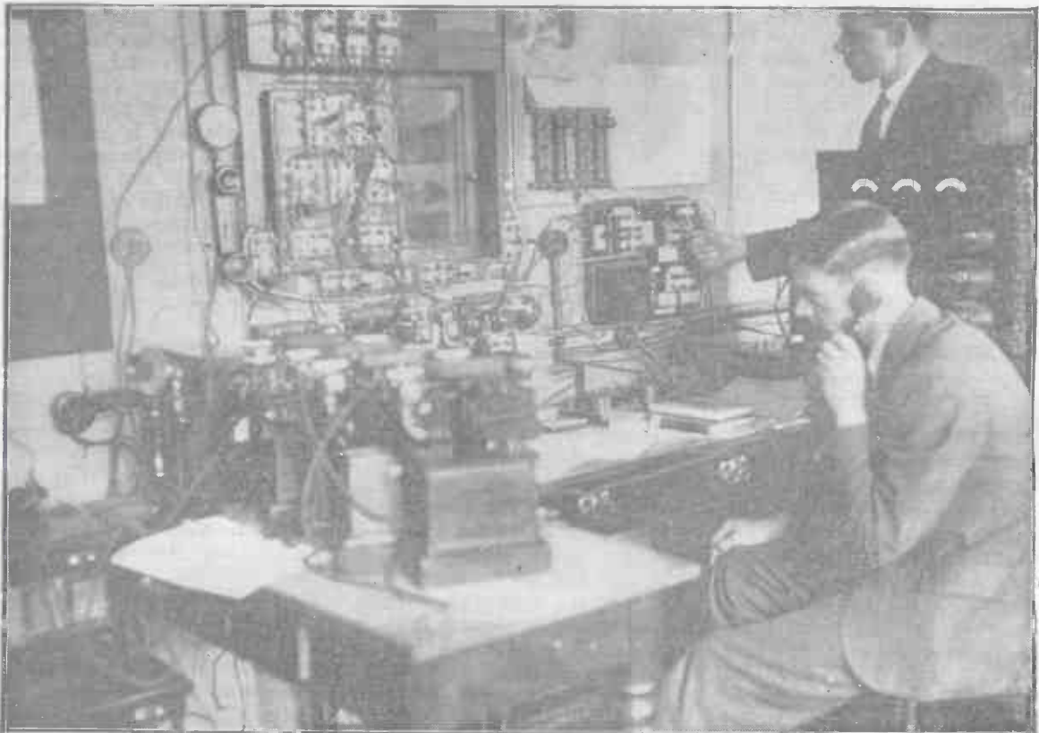
Our photograph shows some of the apparatus at the Glasgow station. The two figures are Mr. L. Holine, the chief engineer (standing), and Mr. H. M. Hill, assistant maintenance engineer.
