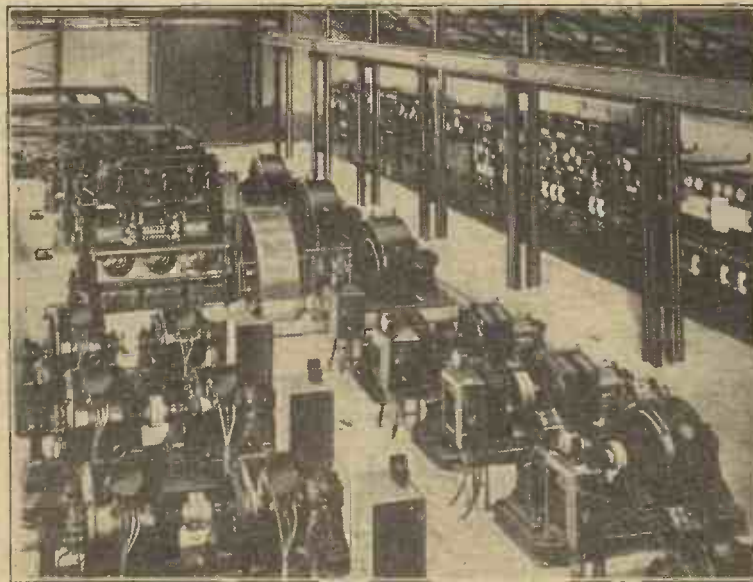
A view of the principal machines in the generator room at the "Beam" station at Bodmin, Cornwall.
