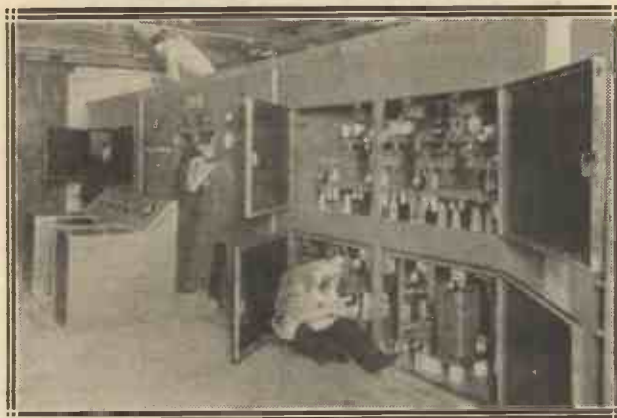
No matter what is done to the transmitter, fading due to the Heaviside layer cannot be completely eliminated, but A.V.C. in the receiver deals with it most effectively. The Marconi broadcasting transmitter being completed above is for use near Jerusalem.
