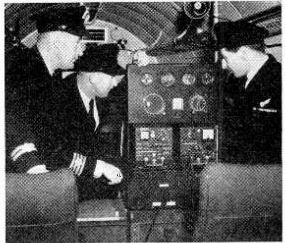
Demonstration AD2300 Doppler navigator installed in a Viking aircraft of Airwork, Ltd.
