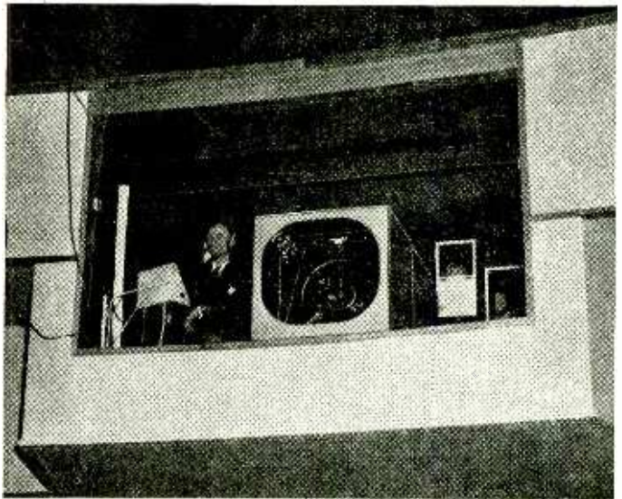
Projection box at the Telekinema seen from the theatre. In the centre is the television projector behind which can be seen one of the two film projection windows. On the left is the transportable television remote-control unit.
