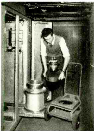
DAVENTRY TRANSMITTER. To facilitate the removal of the high-power valves in the new Marconi air-cooled transmitters, the valve holders are mounted on runners.
