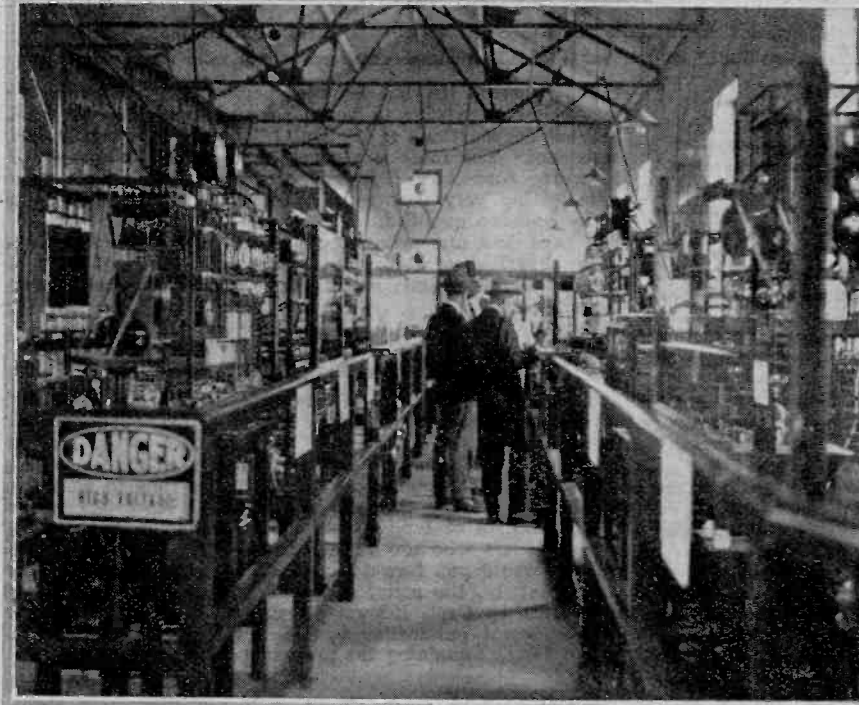
The equipment of the split wave transmitter in which two sets operating on different wavelengths make use of a common aerial. Regular communication with Paris and Burne is maintained.
