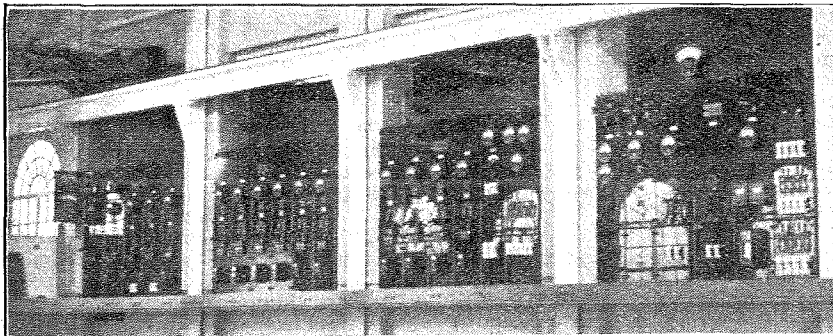
AT HILLMORTON. This glimpse of the switchboard at the new Post Office high-power station at Hillmorton, near Rugby, gives some idea of the magnitude of the work now nearing completion.
