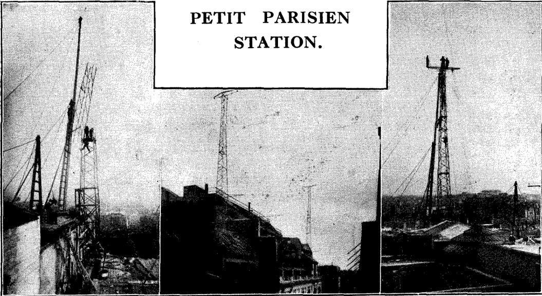
The erection of the aerial masts is shown in the above pictures.
