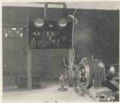
The Dynamo and Switchboard for charging Accumulators.
