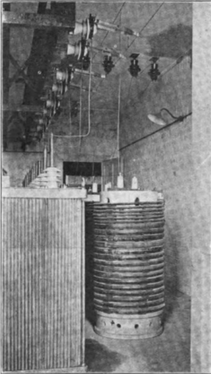
Transformers, Inductances and Isolating Switches.
