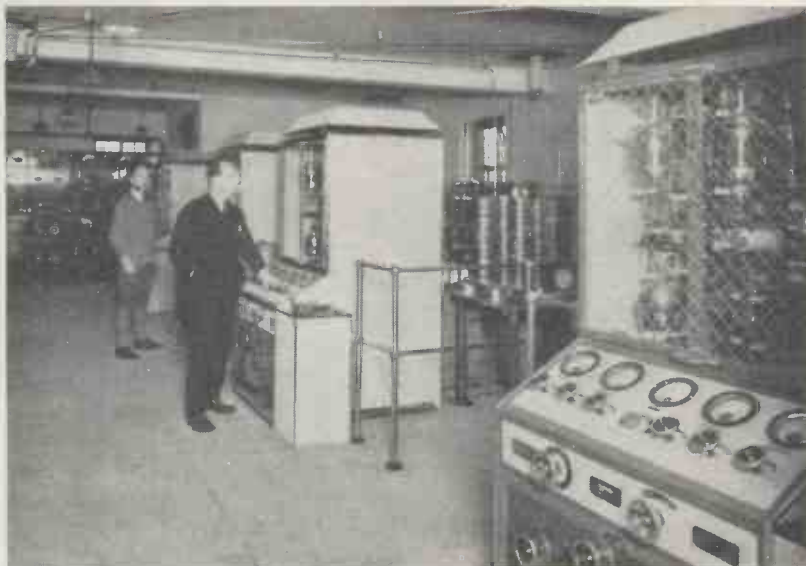
(Left) Compare this installation used at Waddon aerodrome before 1928 with the present up-to-date installation shown in the lower photograph
