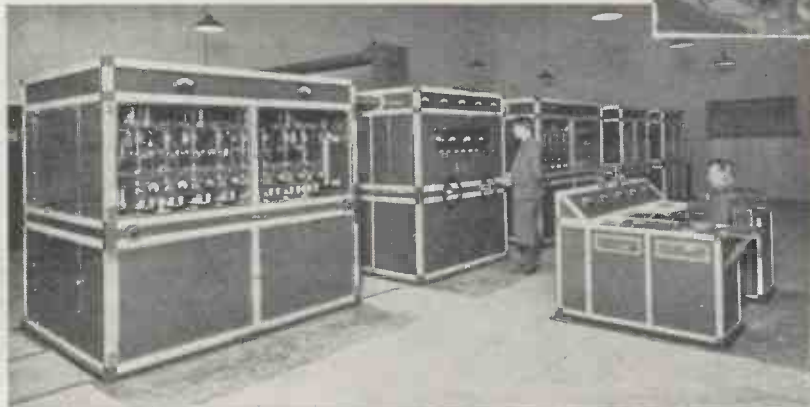
(Above) The latest type of aircraft transmitter as used by Imperial Airways on their Indian and African services. (Left) An example of up-to-date design in broadcast transmitters is shown by this photograph of the Marconi transmitter at the Athlone high-power station in Ireland
