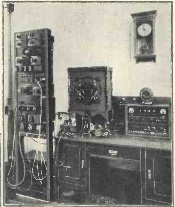
A VIEW OF THE CONTROL ROOM The control room at CT1AA. Note the line amplifier on the left. The studios are about half a mile distant from the transmitter
