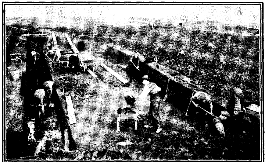
The B.B.C. is making great progress with the new West Regional Station at Washford Cross, near Taunton. This photograph shows workmen excavating for the foundations.
