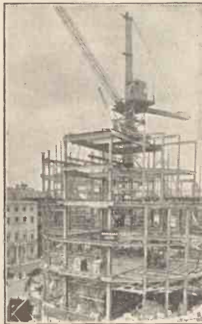
The new B.B.C. building in Portland Place, London, W., is now well advanced, as shown in this recent photograph.
