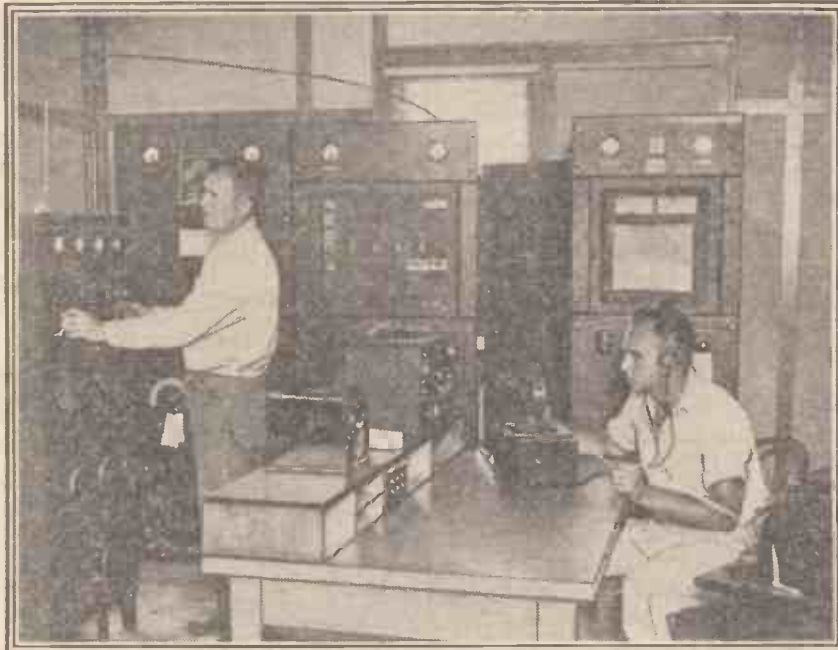
New apparatus installed at Washington for sending, automatically, weather reports to aeroplanes flying on the Atlanta-Boston service. Additionally, this gear will emit a wireless beam for direction-keeping purposes.
