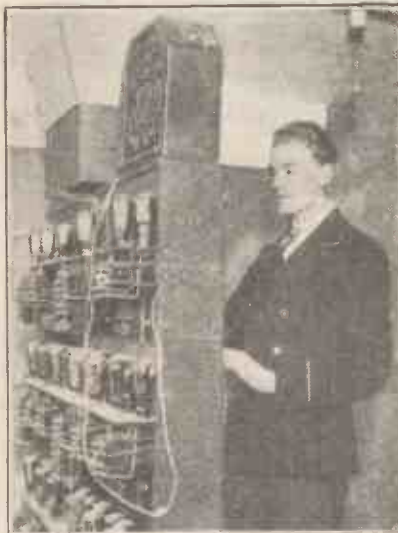
This amplifier, which is used in Baker Street, London, supplies 200 loud speakers. The receiver used in conjunction with it is a three-valver.
