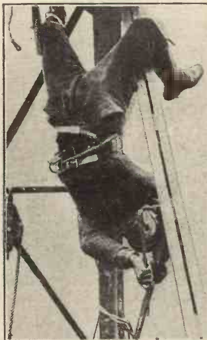
Attitude and Altitude! Suspended high in the air this workman is shown tightening up the mast of the new Langenburg station.
