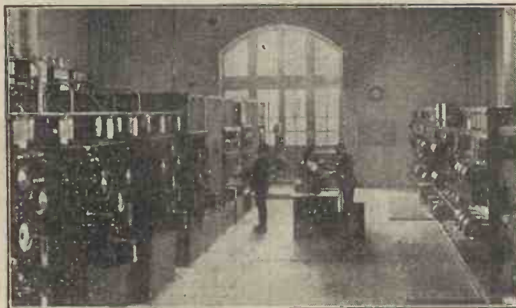
The valve room at Rugby, showing the power units, control tables and switchboard.
