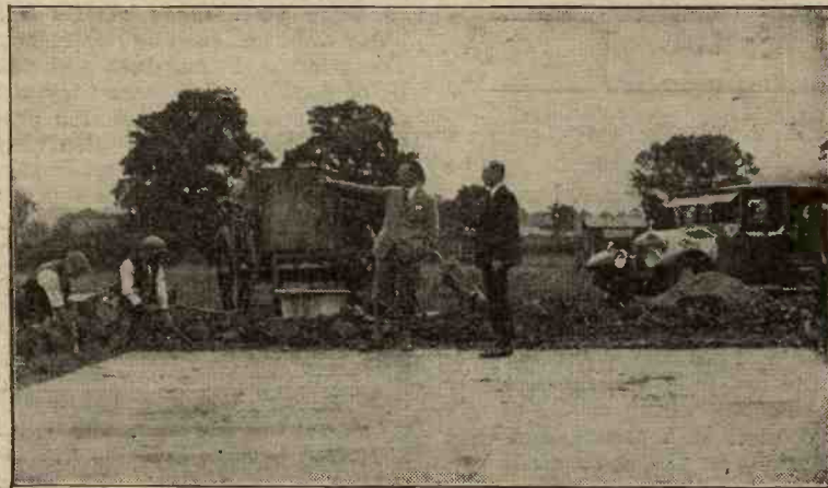
Mr. Scott-Taggart (pointing) and Dr. Robinson inspecting the concrete foundations for one of the buildings at Elstree.
