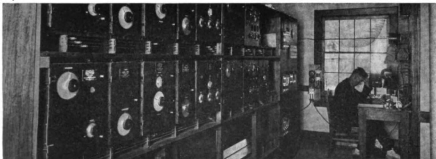
One section of the receiving station. Each shelf contains the apparatus necessary to receive from one European station. Three such sections afford nine receiving circuits
