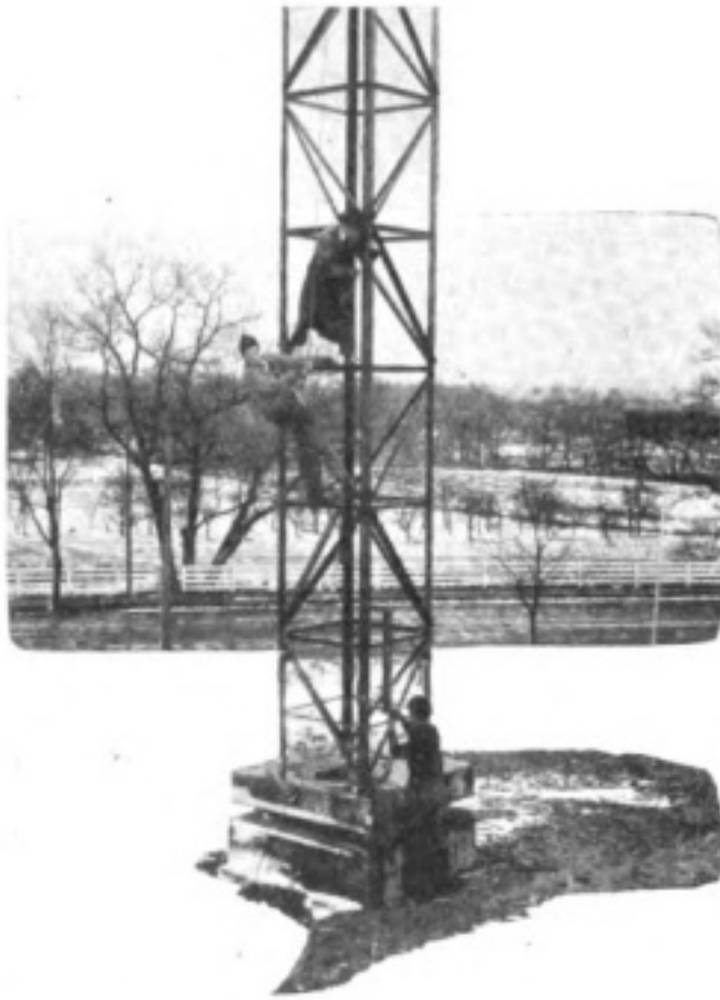
The Tufts tower is supported on four specially designed porcelain insulators which are imbedded in fifteen tons of reinforced concrete.
