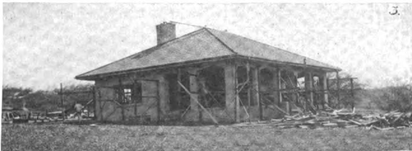
(1) The operating building at the Belmar receiving site is now awaiting the roof tiling, as may be seen in this view taken from the hotel. (2) An illustration of the simple and effective way the mast stays are secured. (3) A typical residence as it nears completion.
