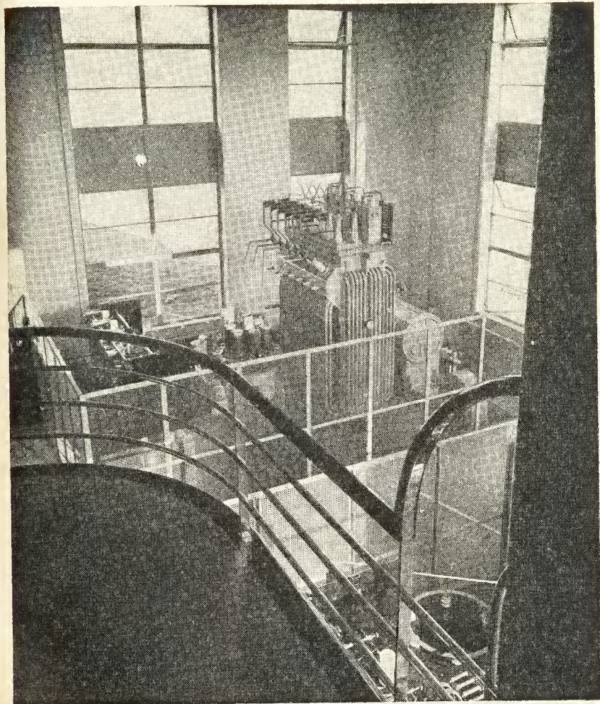
A dramatic view of part of a transmitting station. The large piece of equipment near the corner of the hall is a transformer for one of the mercury-arc rectifiers which provide a high-tension supply at 20,000 volts.
