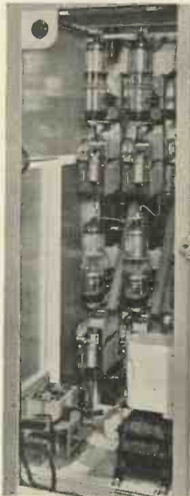
Fig. 5. Rear view of main rectifier
