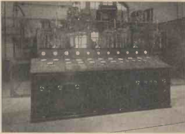
The transatlantic telephone control panel at the Rugby Station.
