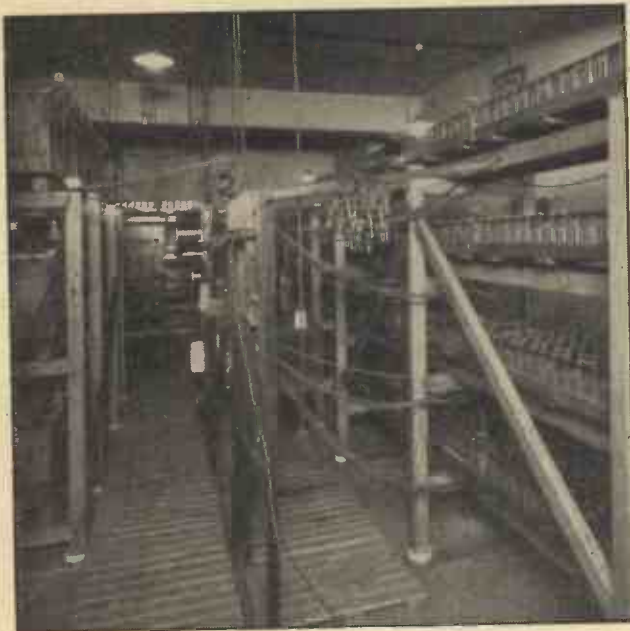
Due attention to the high-tension (and low-tension) supply is paid by the Baird Co., judging by this photograph of a section of their battery room.
