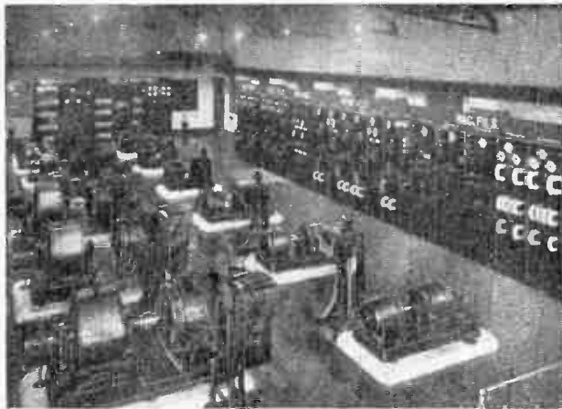
The Machine Room at the Tetney Beam Station.
