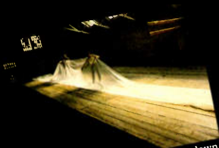
Making the giant water tank. Laying down of the polythene to make the tank waterproof.
