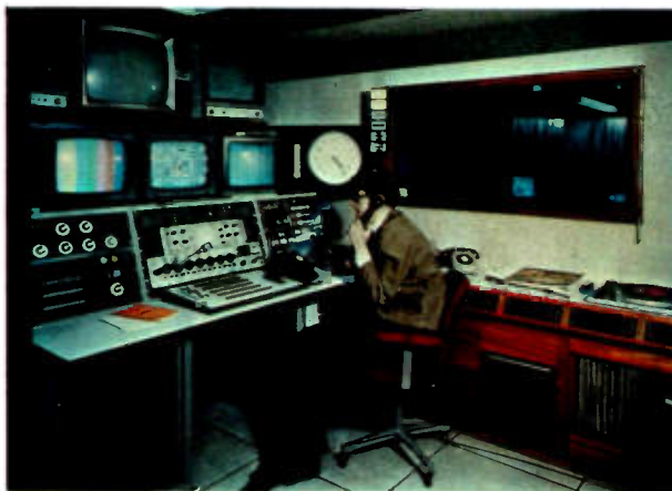
Central Control Room and Colour Viewing Room
