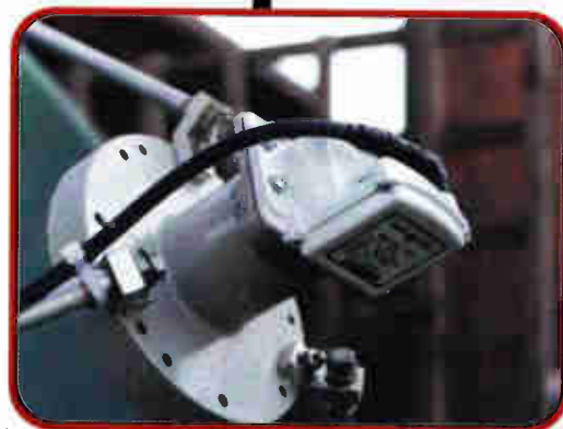
Fig 6: Rear view of my C-Band LNB attached to feedhorn. Note the F-type Plug is carefully wrapped with aluminized tape to ensure waterproof connections.
