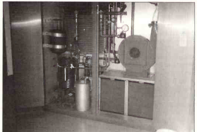
A rear view of the transmitter cooling system - some plumbing!
