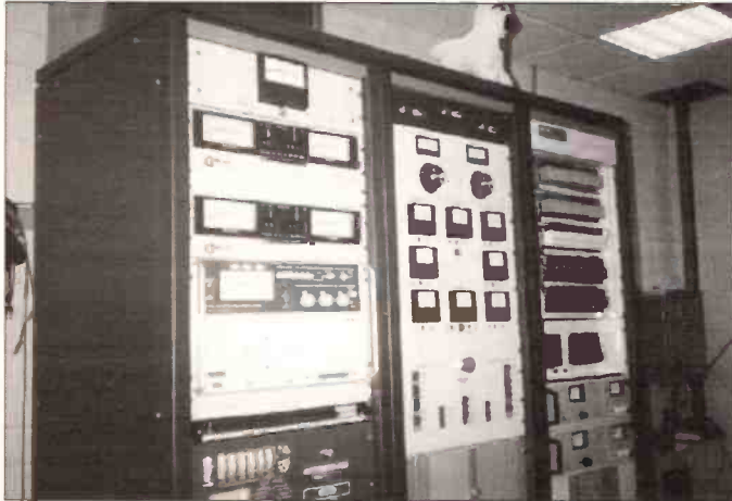
The control room at the Transmitter site, note the 'Atlantic 252' lamb on the middle cabinet. The cabinets contain the test signal generator/distribution analysers and the Optimod processor.
