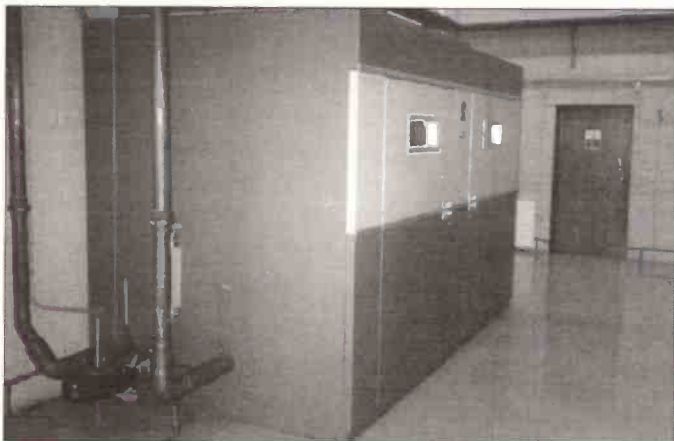
These massive cabinets house the Dummy Load. It is rated at 1MW, to achieve this level of dissipation it is forced cooled by water which circulates at the rate of 726l/m.
