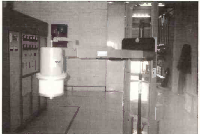
A Thompson TH573 tetrode. Each of the transmitters uses two. They cost a staggering £26000 each!
