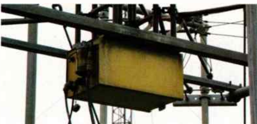
● One of the pneumatic switches used to control the slew of the array.
