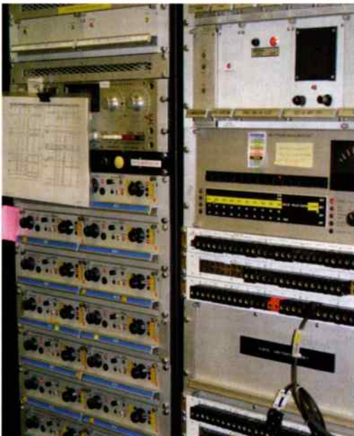
● Woofferton's antenna array control panel. This allows adjustment of slew and forward or backwards radiation.
