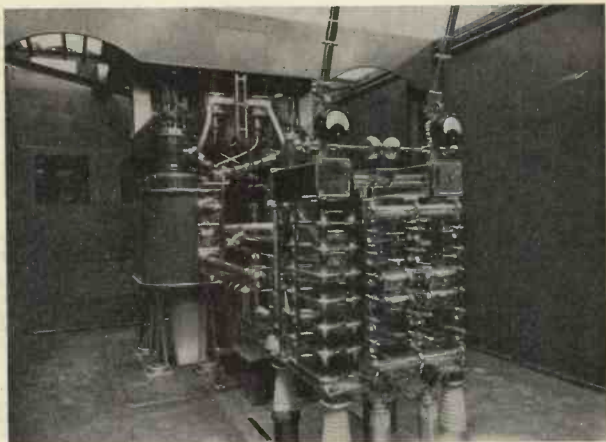
Radio Australia has three high-power short wave transmitters, located at Shepparton (Victoria), 120 miles from Melbourne. This is one of the 100 kW RF amplifiers.
