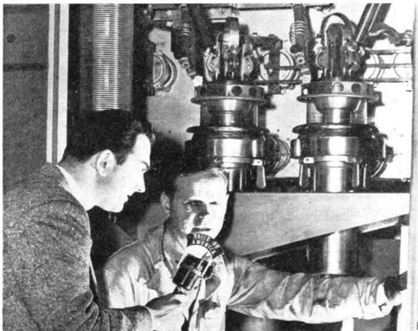
The final amplifier (PA) stage of one of the "Voice of America" transmitters in the broadcasting ship Courier . The engineer-in-charge is recording an explanation of the equipment. The Courier has a world-wide cruising range and carries one 150 kW transmitter and two 25 kW sets.
