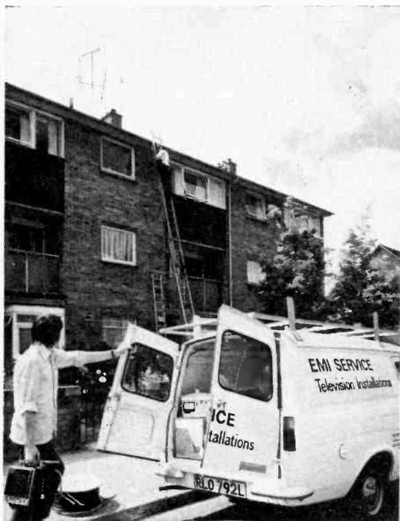
EMI Service will have six mobile installation teams working on the project. The photograph shows one of the teams about to start refurbishing work on a cable television system serving five buildings, containing 32 flats and maisonettes, in Waterloo Road, Uxbridge.
